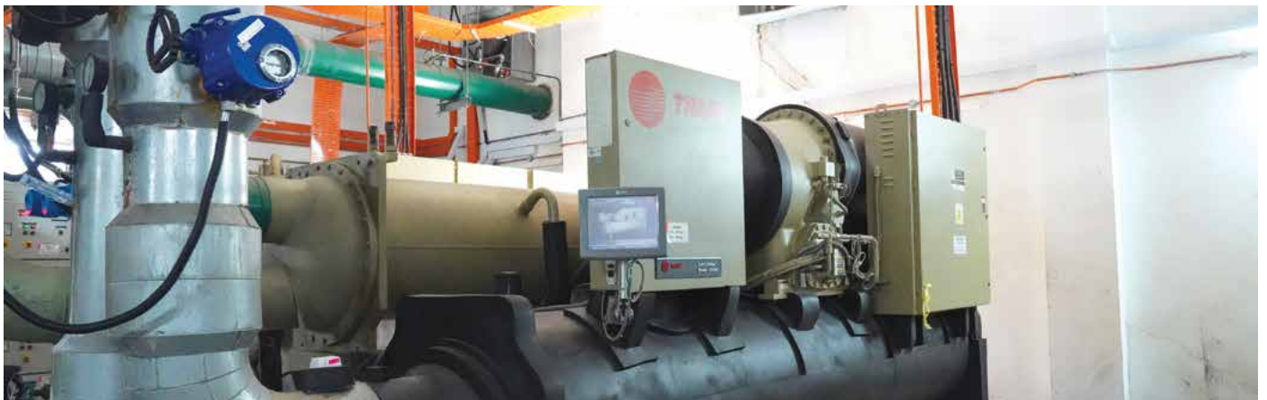
Optimised performance and energy efficiency with Kenanga’s cooling tower fan upgrade
