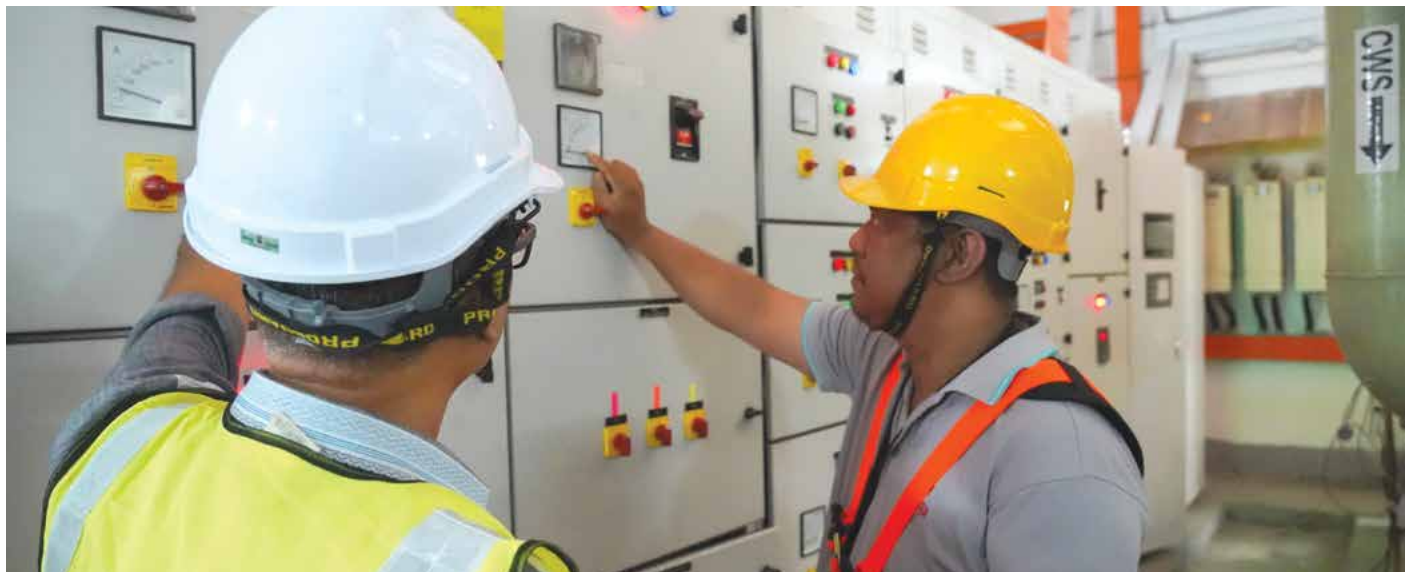
Improved indoor environment control with Kenanga’s advanced sensor integration in HVAC upgrade
