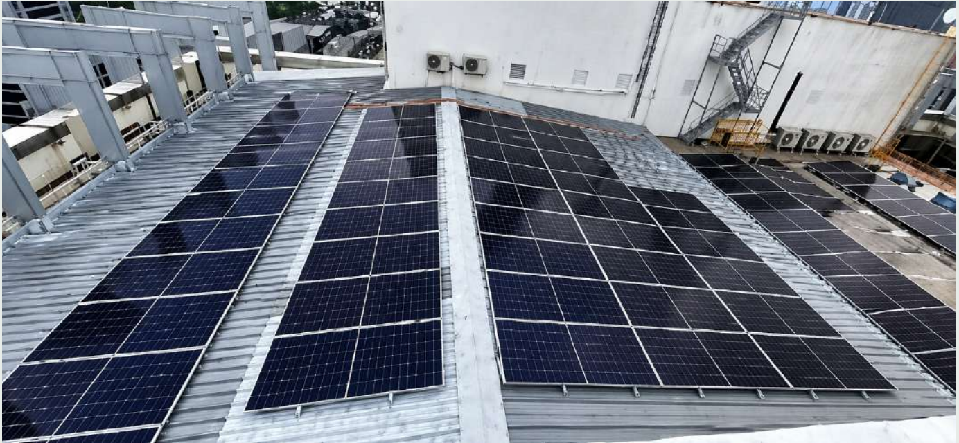
A rooftop solar panel system was installed at Kenanga Tower to increase the share of electricity sourced from renewable energy, supporting our efforts to decarbonise Scope 2 emissions under the Decarbonisation Roadmap.
