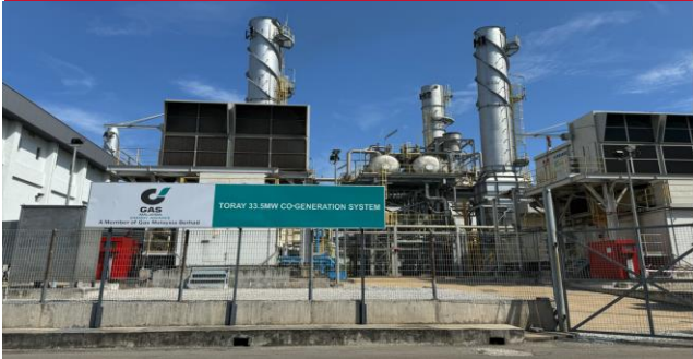
Exhibit 1: Toray Cogeneration Plant
