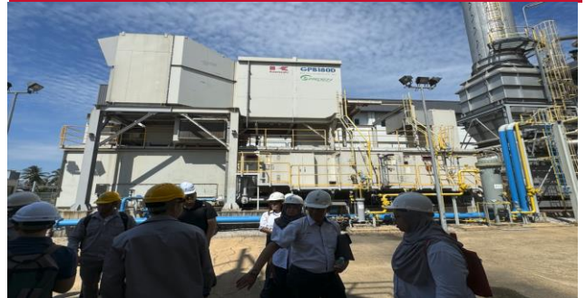
Exhibit 4: Gas Turbine Generation Set
