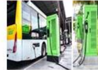
Charging stations for our electric buses
